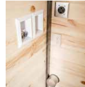
WASHER & DRYER HOOKUPS
