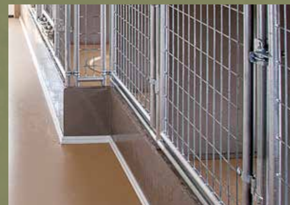
Interior Raised Floor
