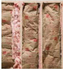
R-13 Batten Insulation In Walls & Ceiling
