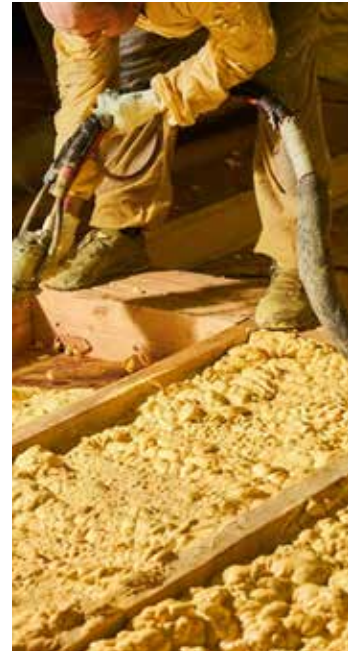
Spray Foam Insulated Floor
